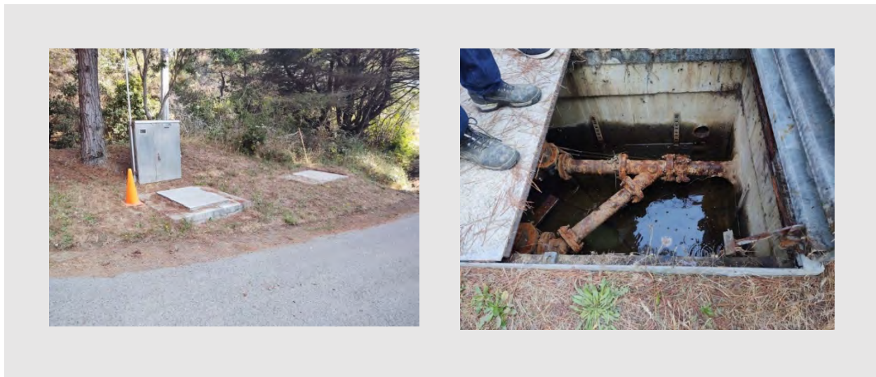
Figure 2.4.2-1 Lift Station 1 from Street and Under Hatch
