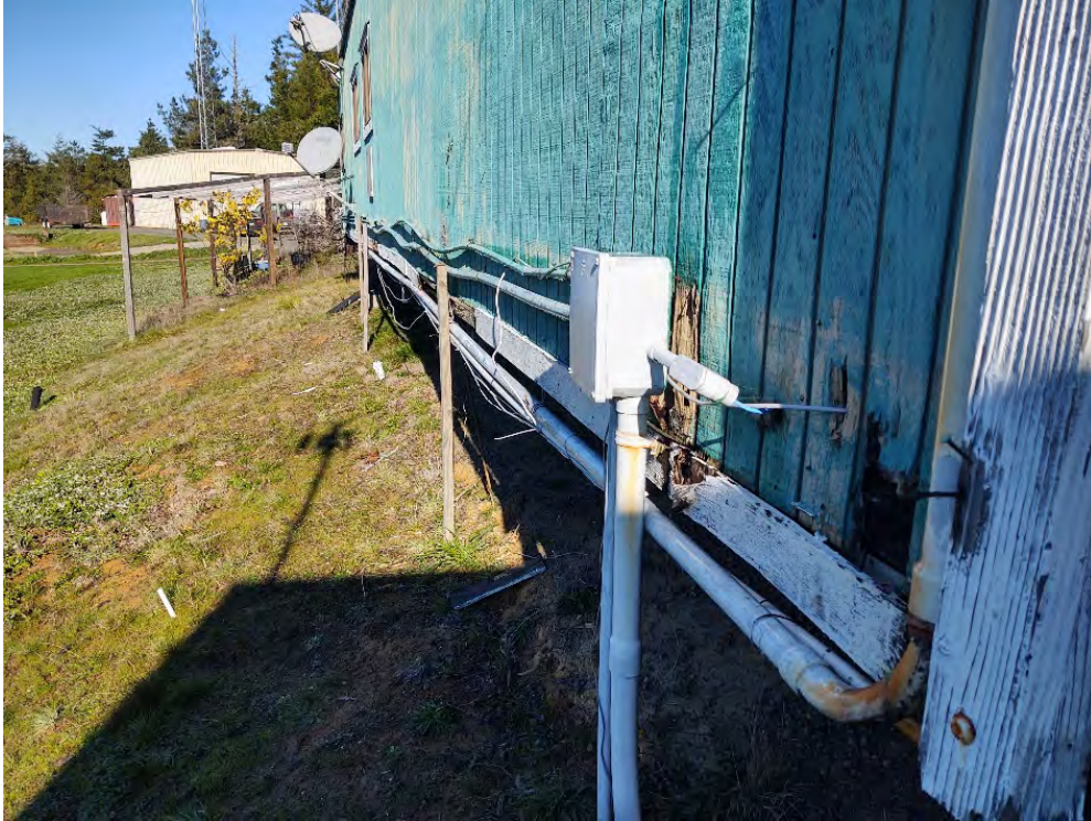
Figure 5.3.1-2 Existing Administration Building Deterioration
